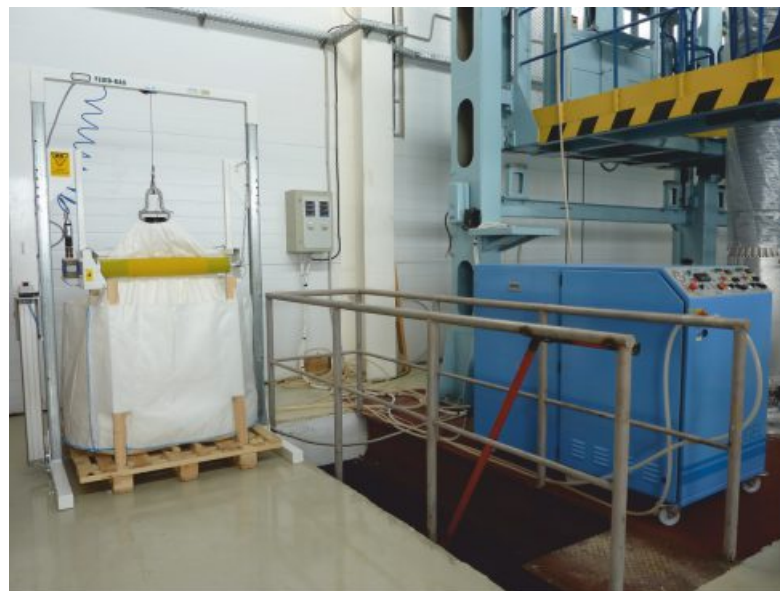
Fig. 20 Unit for degassing and metering feed of compression gel at Izolyator plant
